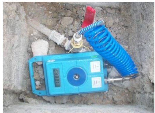
Data logger Fixed During the Establishment of DMA to measure the water loss in the DMA
