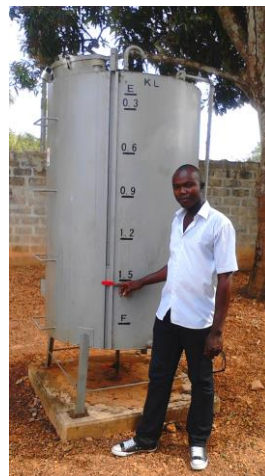
Fuel tank gage showing fuel supply to water treatment plant
