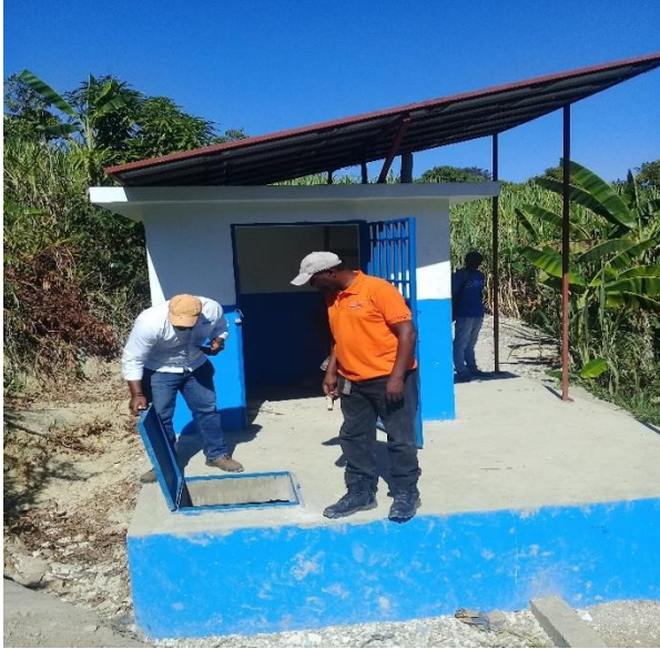
Grand Boucan – Water system with solar pump
