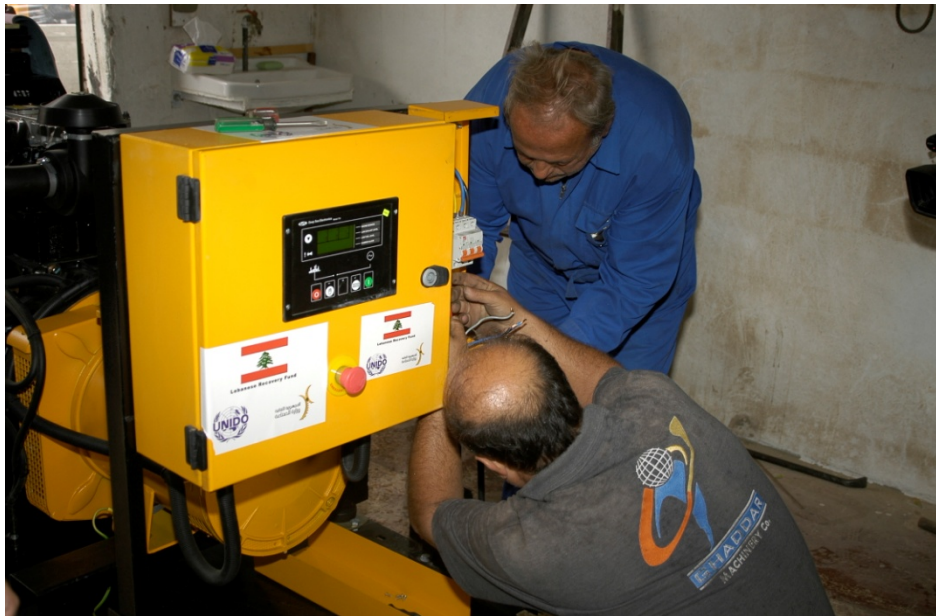
Provision of new generator, Abou Ghida, Kham
