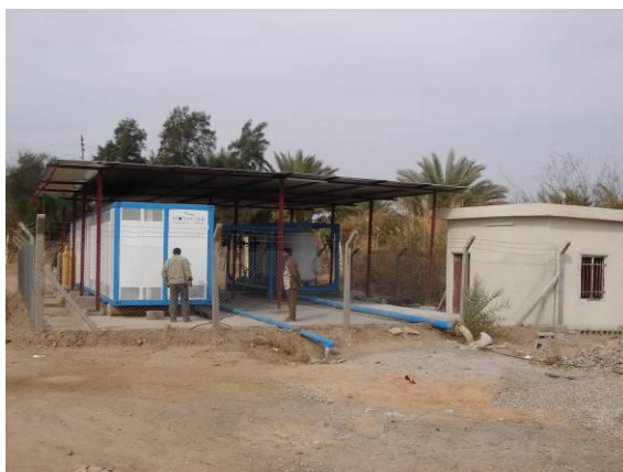
Rehabilitated Compact Unit in Al Mansya, Wassit governorate
