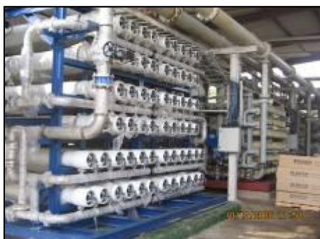
Newly installed RO Skid
