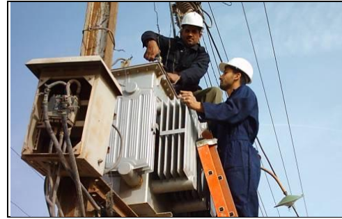
UNDP power generation project 2009
