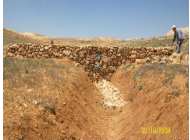
Stone walls for runoff interception
