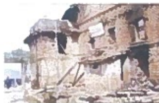
Fig.: Destroyed Office Building in Achham
