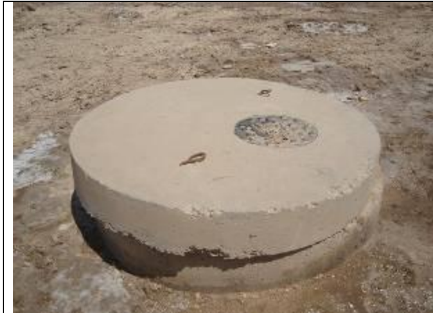
Samawa /Supply material and construct a storm water network at Al-Askri - RCFI/SA/W05
