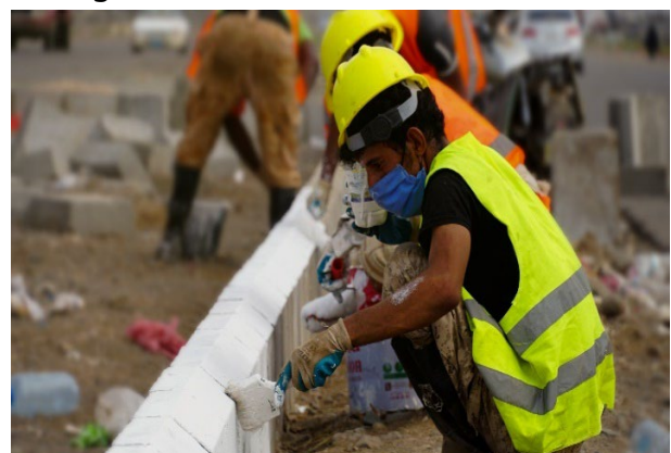
Part of road rehabilitation in Lahj to ease communities access to markets, 2021
