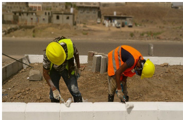
Part of road rehabilitation in Lahj to ease communities access to markets, 2021
