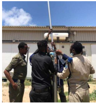
SPF communications engineers install antennae for the tactical radio system in a JOC
