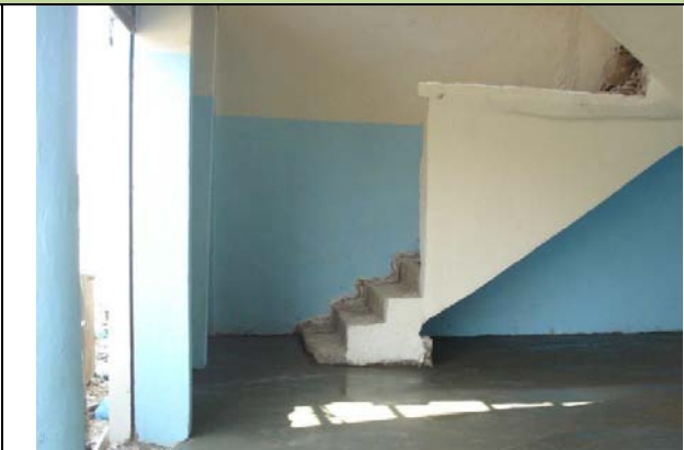
The surfaces such as the walls and stairs have been renovated and painted in two different colors.
