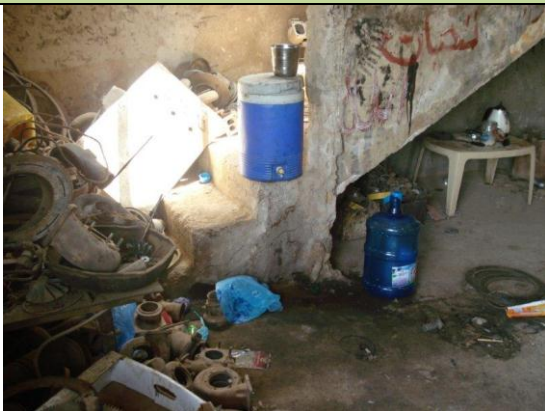
The stairs, walls and floors at Majeed Workshop are in very bad condition.
