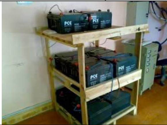
Al Fadhelah school- ICT facility / battery
