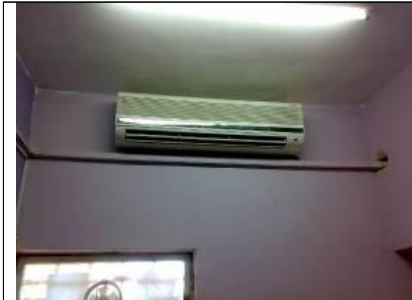
ICTDC centre-one of the supplied air cooler
