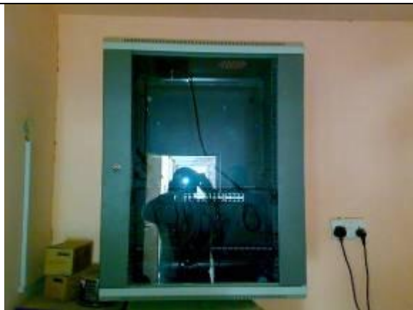
Al Fadhelah school- ICT facility / Server
