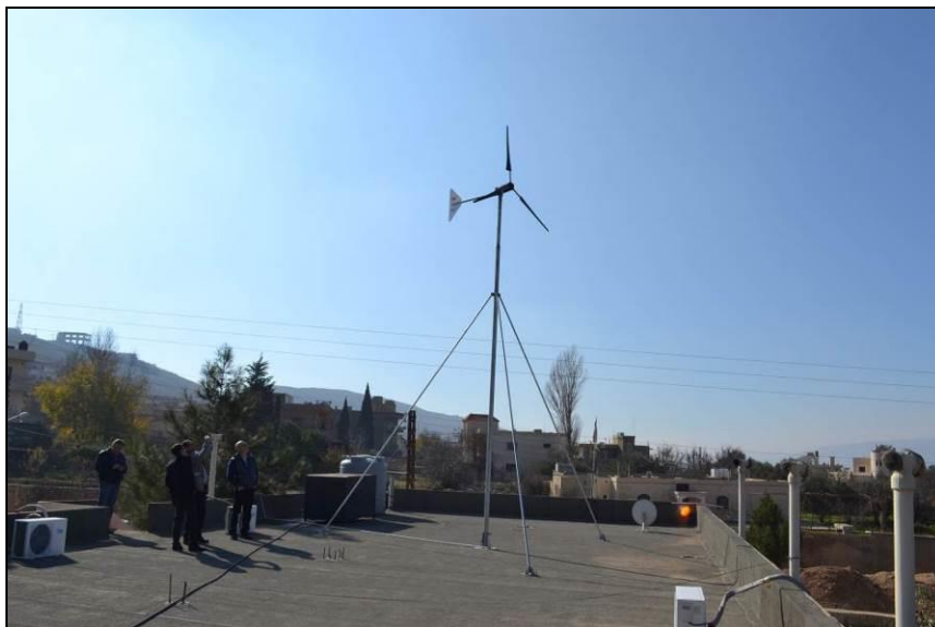
Microwind Turbine in Ras Baalbeck Community Center
