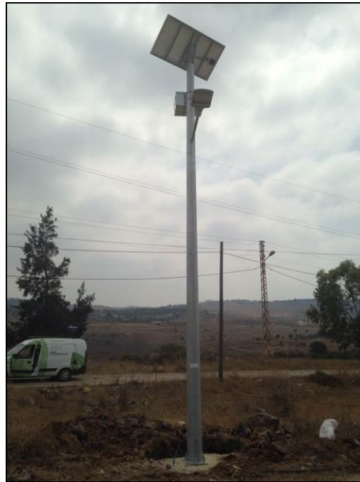
Solar Street Lighting - Menjez
