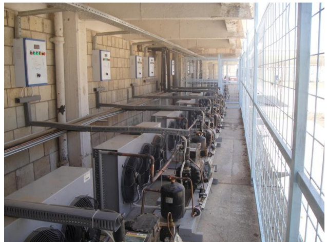
new battery of compressors for cooling
