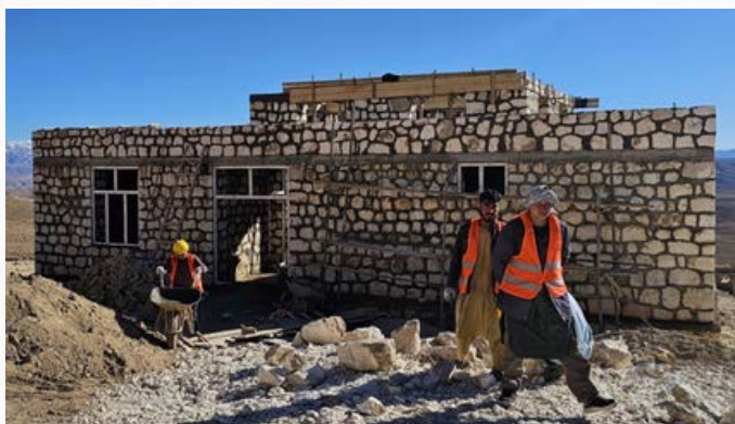
The final stages of construction of a FHH underway in Charcheshma village. Photo: IOM 2024
