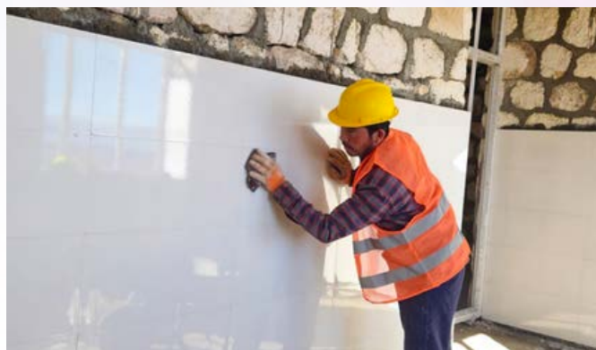
A worker cleans tiles as part of finishing works at an FHH in Charcheshma village. Photo: IOM 2024
