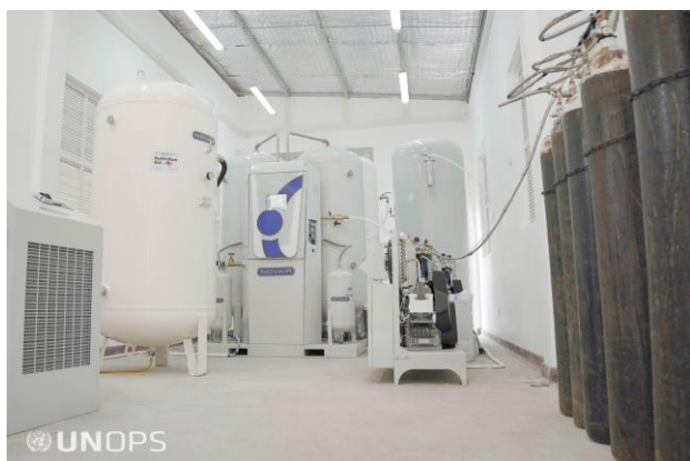
Oxygen Plant, Mullaitivu District General Hospital
