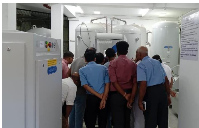
Oxygen Plant, Polonnaruwa District Hospital
