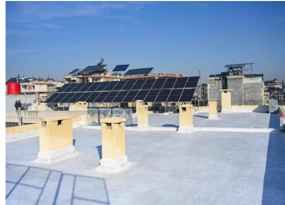
Figure 12- Midwifery school rooftop, solar panels.
