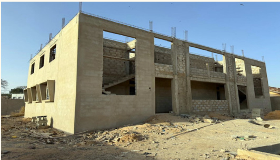
Construction of a daycare facility for the Senegal National Police, Thiès, Senegal, December 2025.
