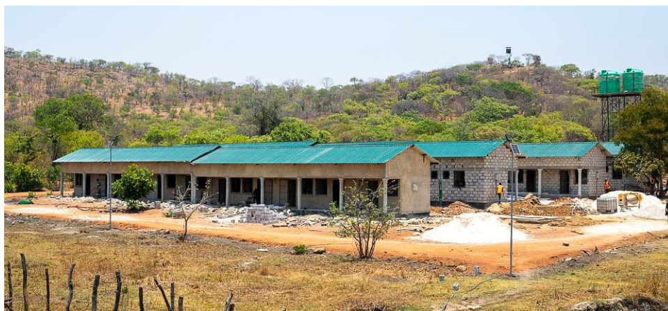
Construction of the 40-bed accommodation block and daycare facility for women police officers, Zambia, 2025.
