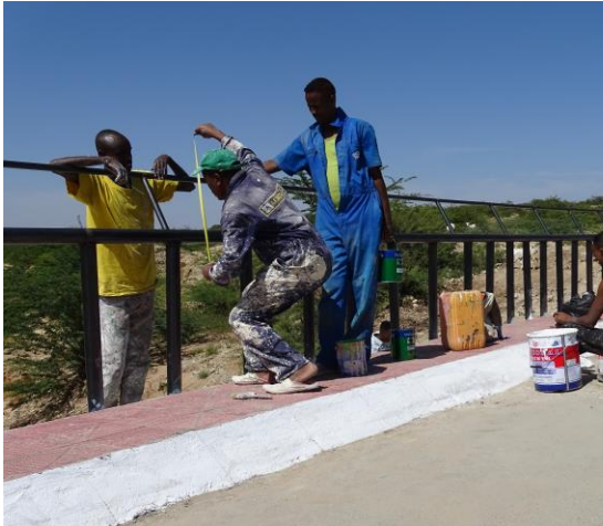
Finishing up on East and West Gabiley Culvert Box and Access Road, with support from the Local Development Fund, October 2017
