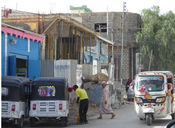
Construction on the side of a new tarmac road with Bajaaj parked outside a shop, October 2017
