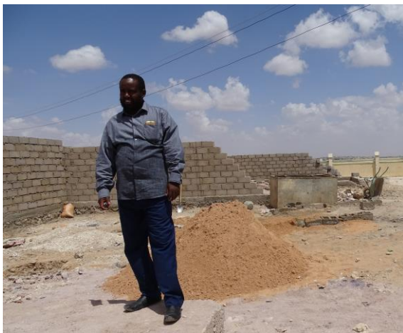
Asha's Engineer at the Kodbur fire station construction site in Hargeisa, where building is underway, October 2017
