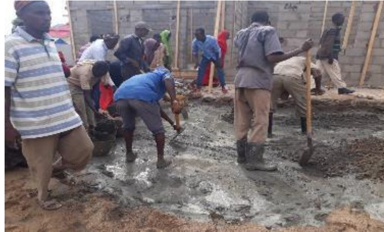
Cash-for-work beneficiaries participate in the construction of Aqoon Side Primary School in Kismayo District © Omar Salad Mohamed / UN Migration Agency (IOM) 2017
