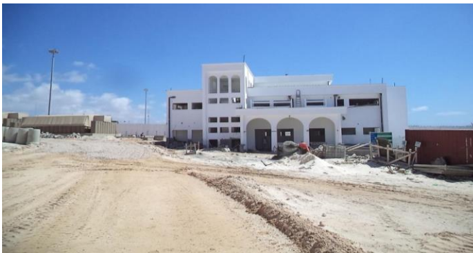
Mogadishu, December 2020: Electoral Dispute Resolution Centre under construction at new NIEC compound.
