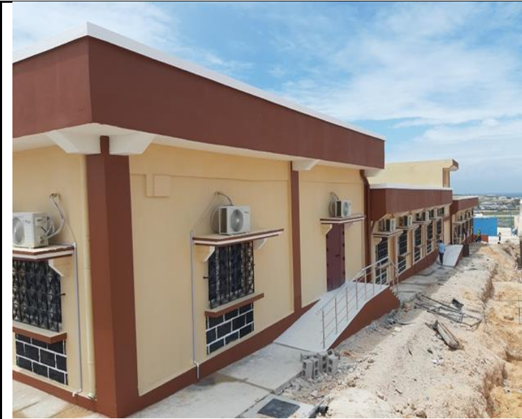
NIEC Data Center Building, NIEC compound, Mogadishu, May 2020
