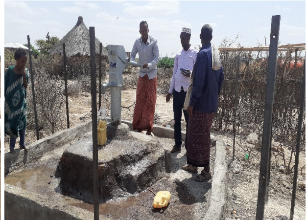
Dalada kebele rehabilitated hand dug well
